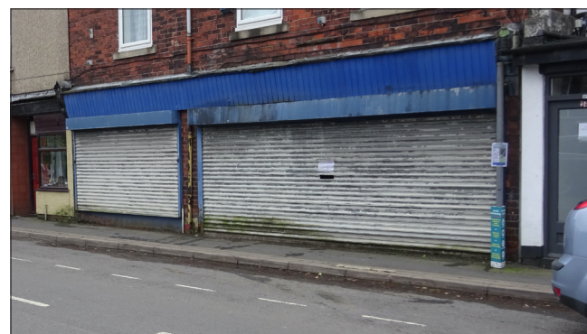
Unattractive shop front shutters
