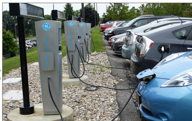
Electric Car Charging Station
