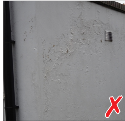
Portland cement based renders. These do not allow the building to breath and when cracks appear, water ingress can severely damage the building fabric.
