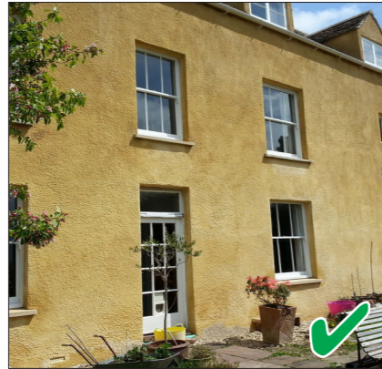
Traditional lime mortar which is breathable and flexible. Here it's finished with a coloured lime wash.
