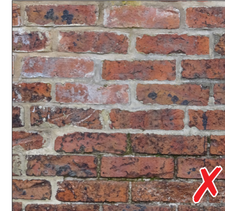
Repair work: mismatch in brick colour and bad pointing. The whole wall needs to be considered as this will never match-in over time.
