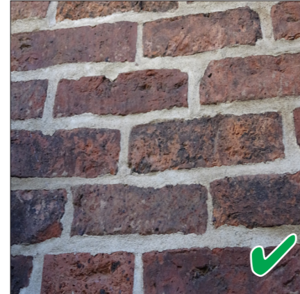
Many styles of pointing have evolved over the years but few are acceptable in the Conservation Area. Flush or nearly flush is the desired look for the Conservation Area in Tibshelf.
